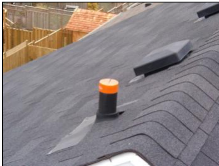
18. Plumbing stack is capped
