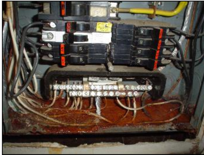
6. Water and rust in bottom of panel
