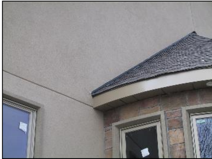
1. No kickout flashing at roof/sidewall junction
