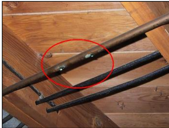
16. Leaking copper supply pipe
