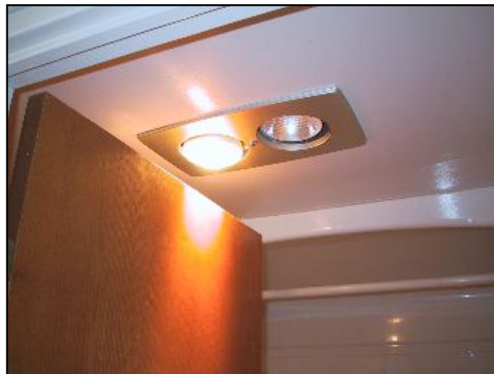
8. Heat lamp over door - fire hazard!
