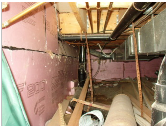
15. Exposed polystyrene insulation is fire hazard
