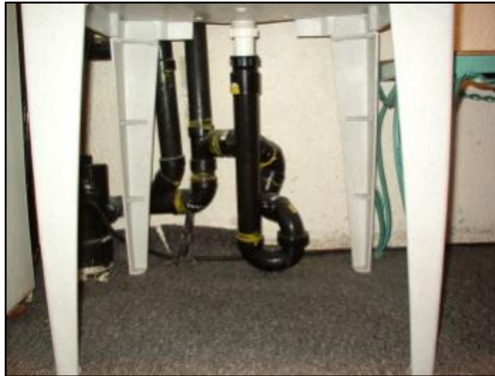
17. Poor trap arrangement
