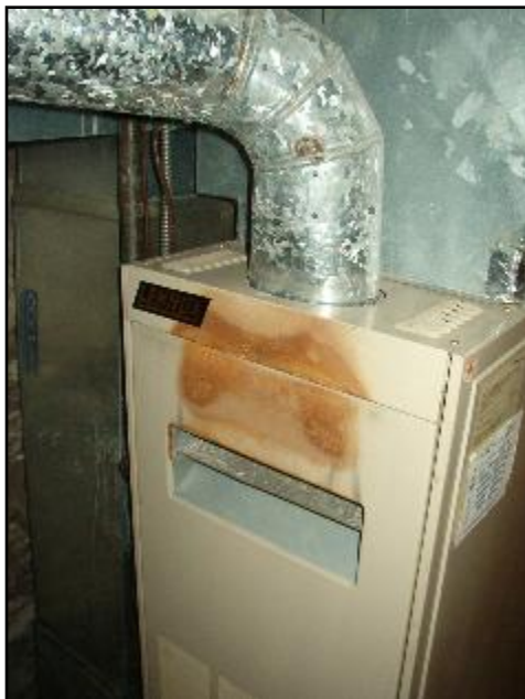
9. Evidence of furnace backdrafting
