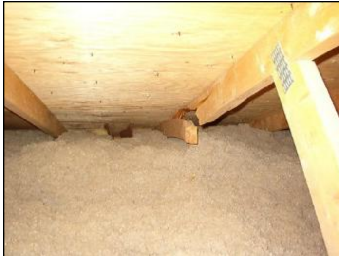
5. Top chord of truss is broken
