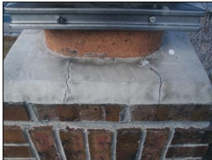
12. Minor cracks in chimney cap
