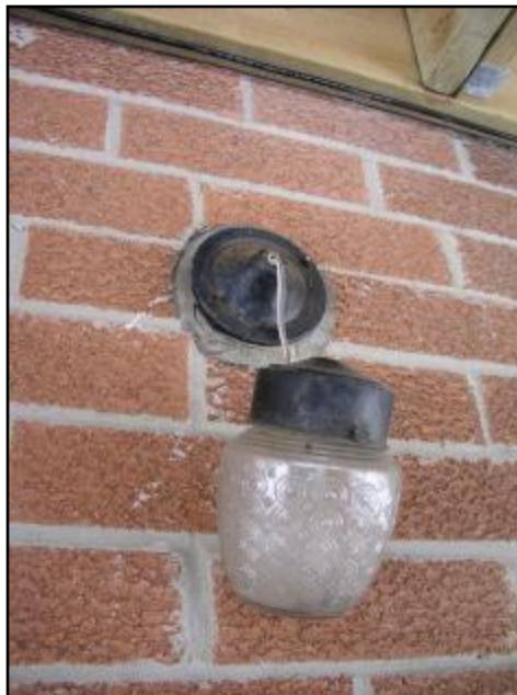
7. Light fixture is not well secured
