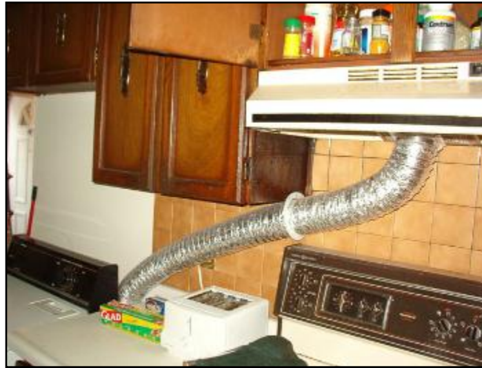
22. Clothes dryer vented incorrectly
